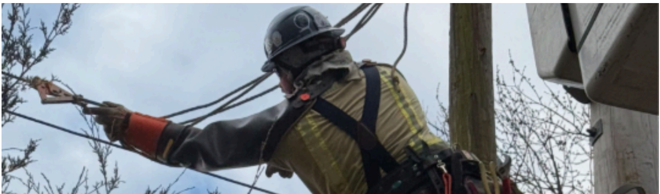
Various Electric Department project around the village.
